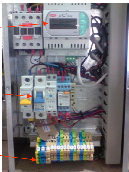
Fig 13 Electrics box with the front removed
