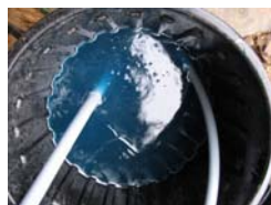
Fig 24 Slinkies Purged of Air
